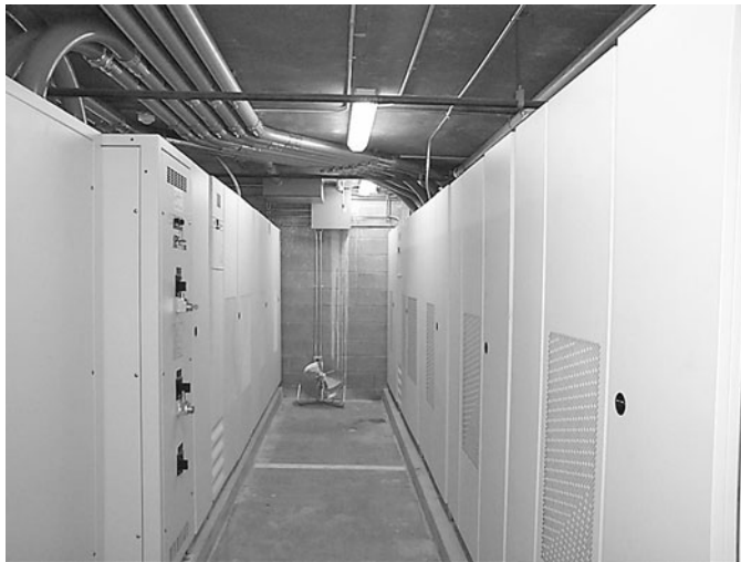
Figure 6.1 A modular UPS at GNAC, Inc.
