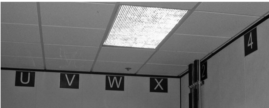
Figure 6.8 Numbering high on the walls of the data center in Synopsis is used for rack naming and makes it easy to locate a given rack.
