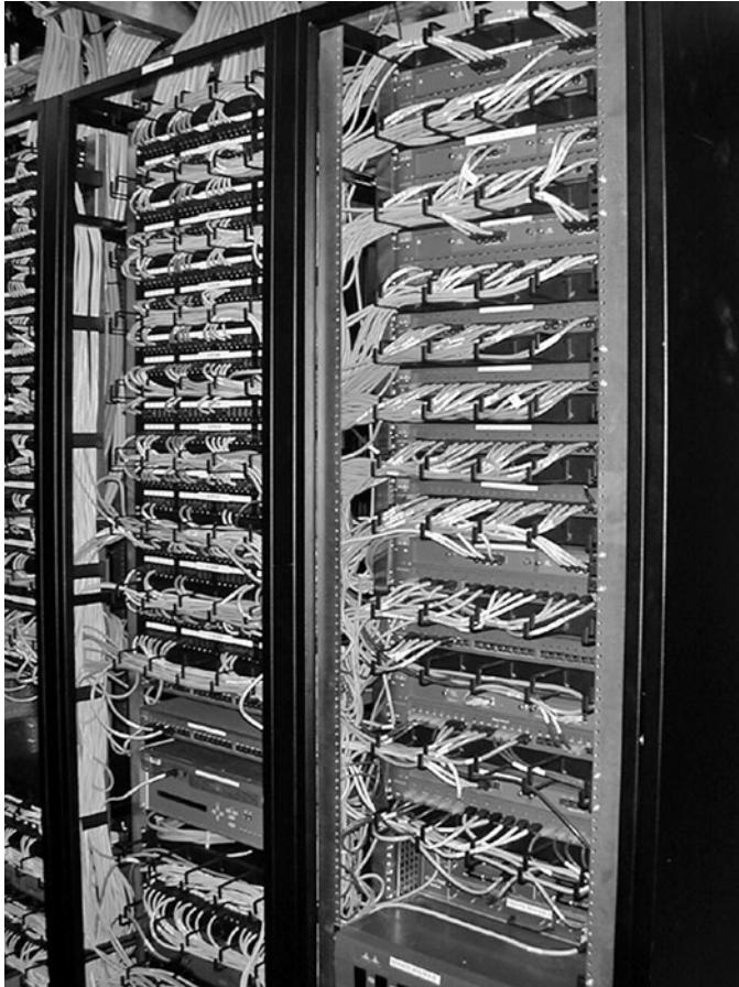
Figure 6.11 Network racks at GNAC, Inc. (Patch panels are connected to overhead cabling to prewired patch panels at the top of each host rack.)
